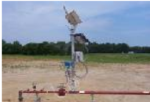
Plate 1: Production Field Installation - Solar Powered Battery Backed System.
