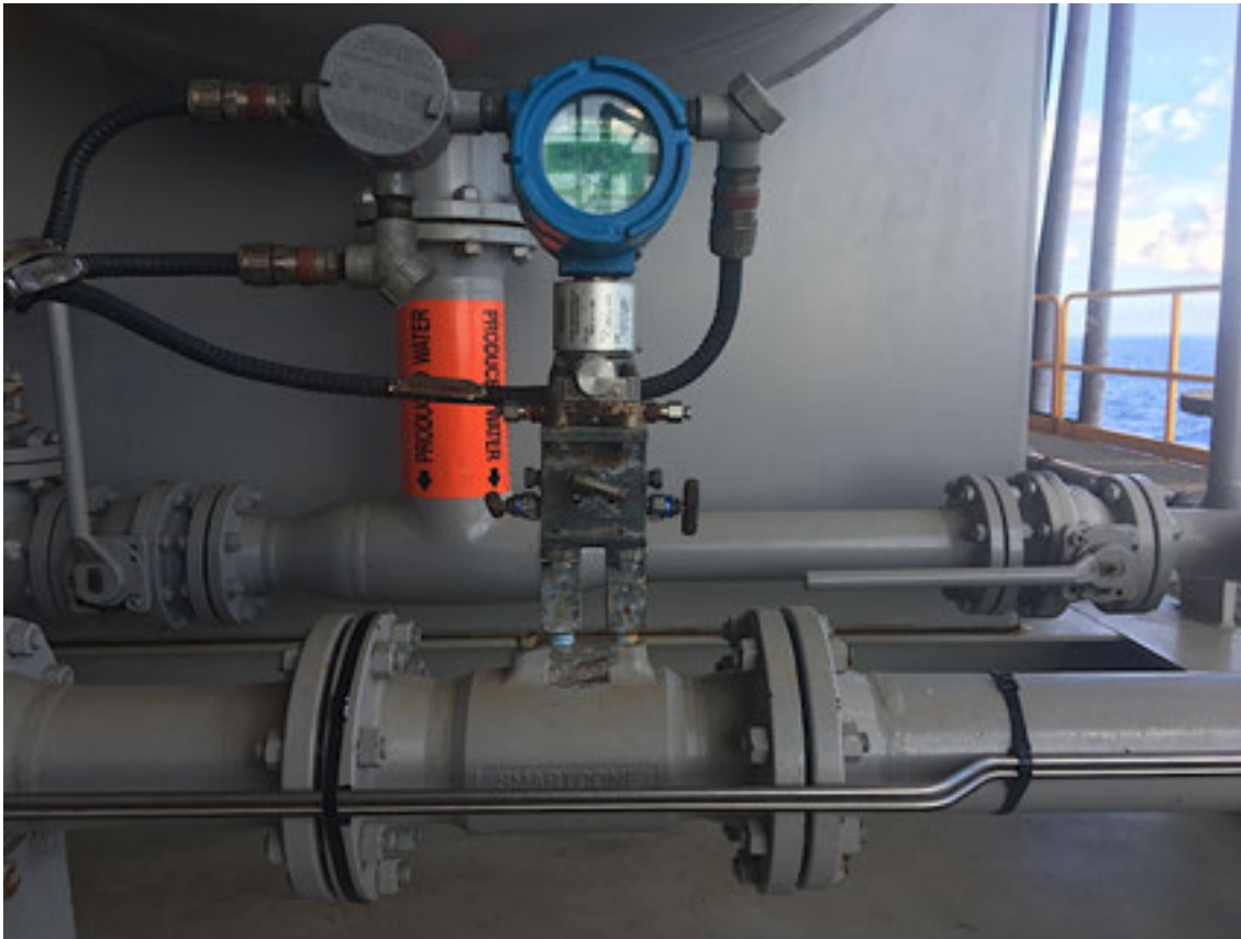
Walter Oil and Gas - Offshore Platform Produced Water Measurement
